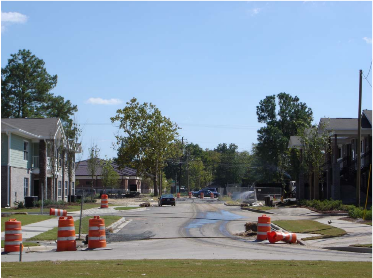
September 28 – Peabody Site - view along the new Midland Street looking toward Talbotton Road from the traffic circle. Ready for final paving to complete connection to Talbotton Road.
