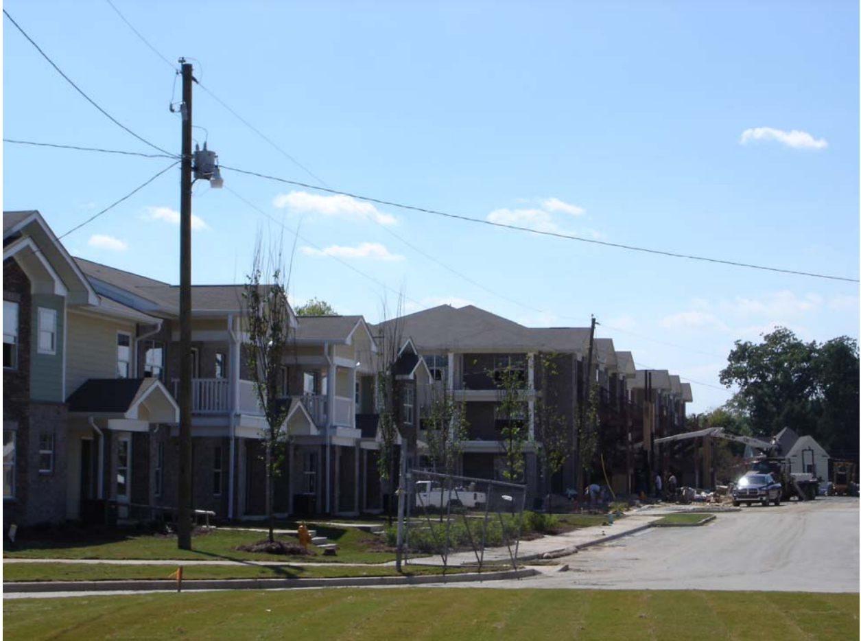
September 28 – Peabody Site - view along the new Olive Street from the traffic circle. Getting ready to complete paving. Building 19 at left with Building 10 and 11 beyond
