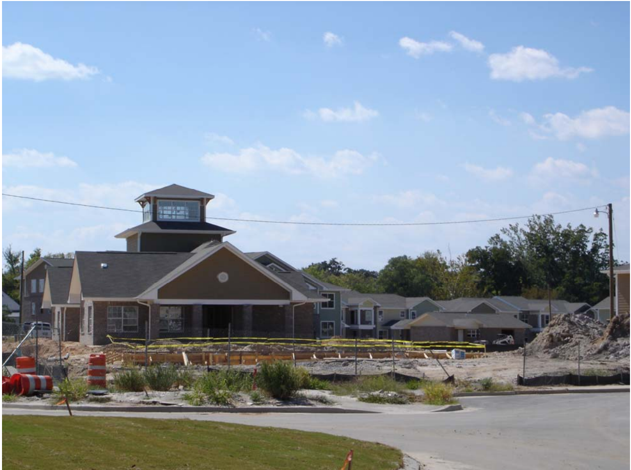
September 28 – Management Office - view from traffic circle – swimming pool under construction in front of the building.
