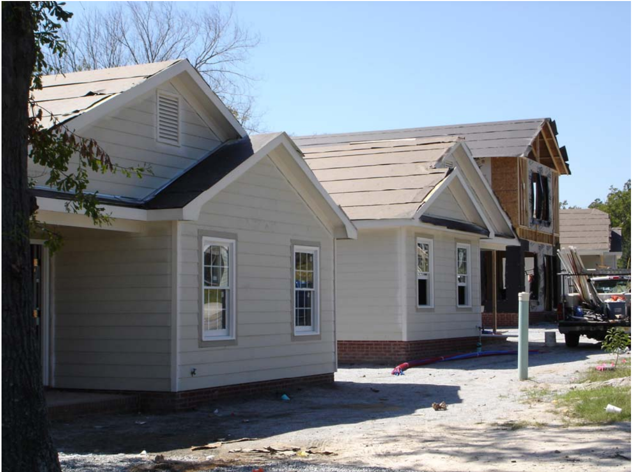
September 28 – E Wynnton Phase 1– 9 Home Program south side of 8 th Street – Buildings 1, 2, 3, 4 under construction.
