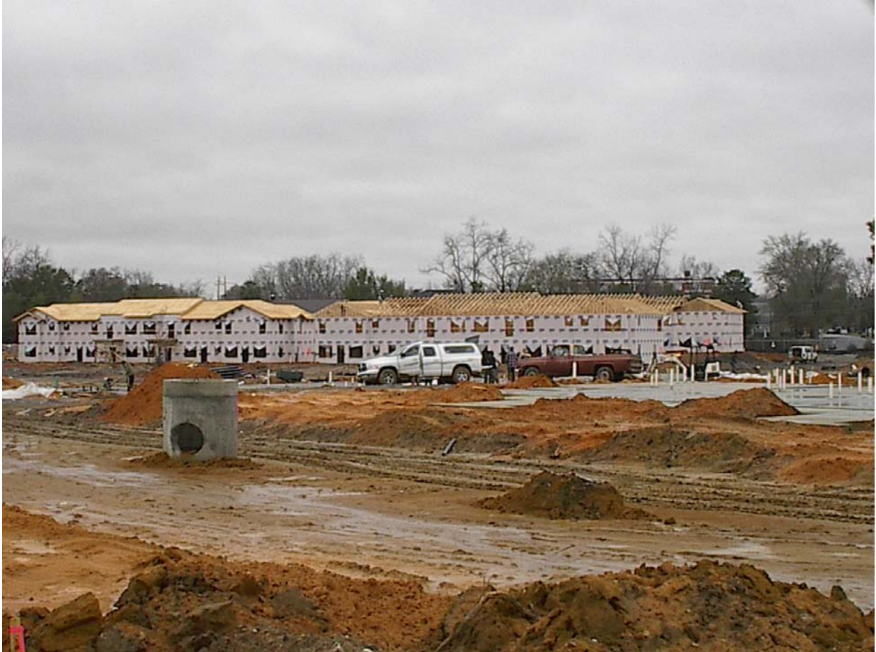
02-02-06 view looking northerly across the site. The new 11 th Avenue in the foreground, Buildings 15, 16, 17 and 18 in construction in the background.
