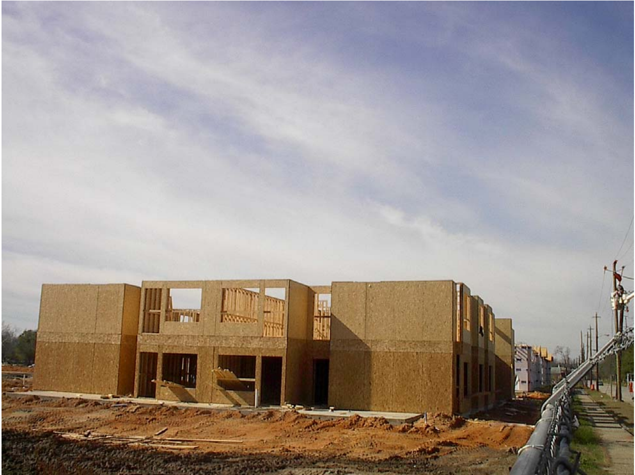
02-01-06 view of new building construction. Looking westerly along 27 th Street at Building #1 from the east. Georgia Power at right side making revisions to existing overhead power services on 27 th Street.
