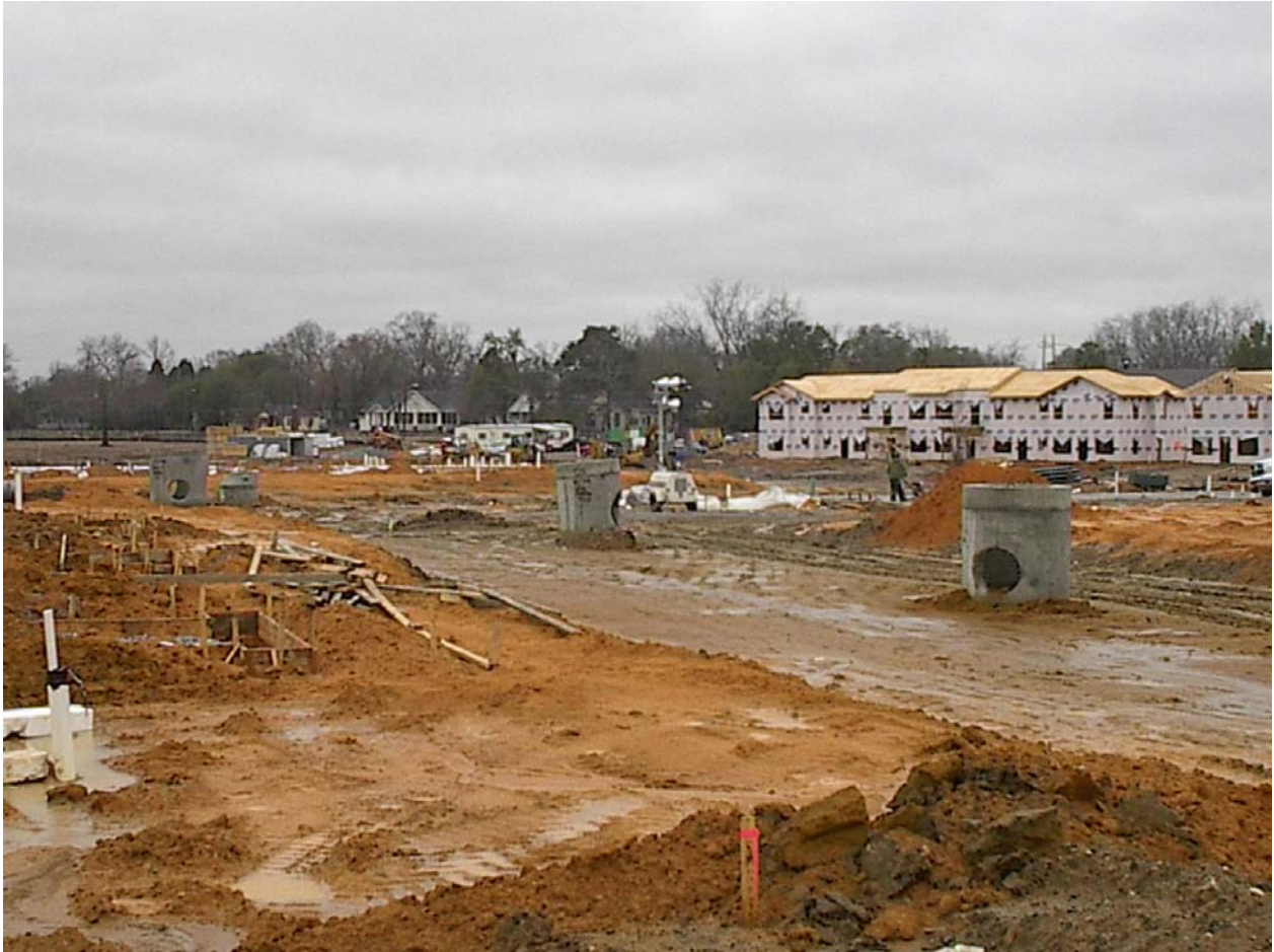
02-02-06 view looking northwesterly across the work area from Ivy Avenue. The new 11th Avenue from Talbotton Road in the foreground.
