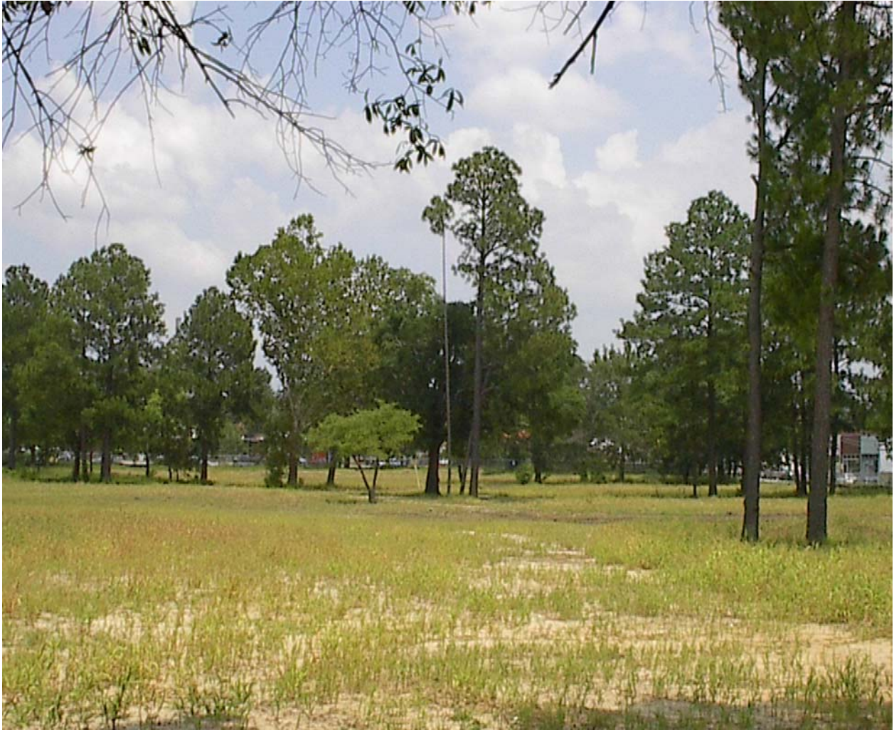
08-03-05 Demo Phase 1 Site Area – looking easterly toward the future Phase 3 Development site area from existing Ivy Avenue
